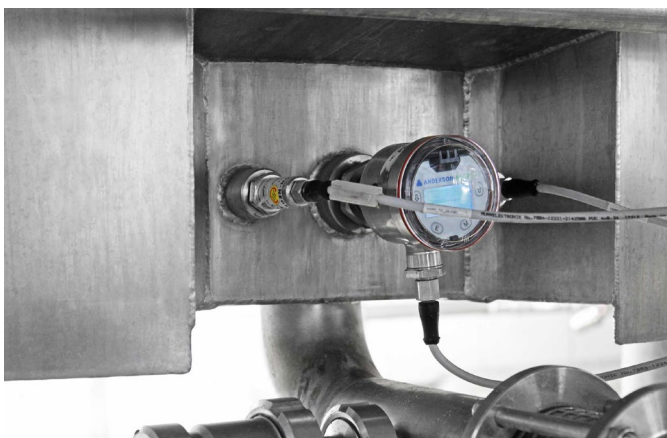
Common practice for storage and maturation tanks: Simple installation of hydrostatic level sensor (here L3 Neo), temperature sensor and point level switch on the underside of the tank
