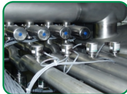
Fig. 3: Flow monitor, type FWA-141, built into the return for monitoring the CIP circuit.
