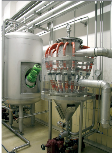
Fig. 1: Left: Storage tank for the tartar seed crystals Front: Venturi centrifuge
