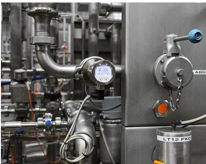
ITM-51 for the control of the blowdown of the spent yeast
