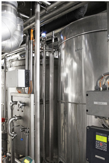
Maturing tank for biological acidification with level meter NSL-F in the riser tube
