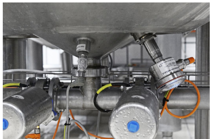
Monitoring of the CIP tank for membrane filtration with TFP temperature sensor and L3 pressure and level sensor
