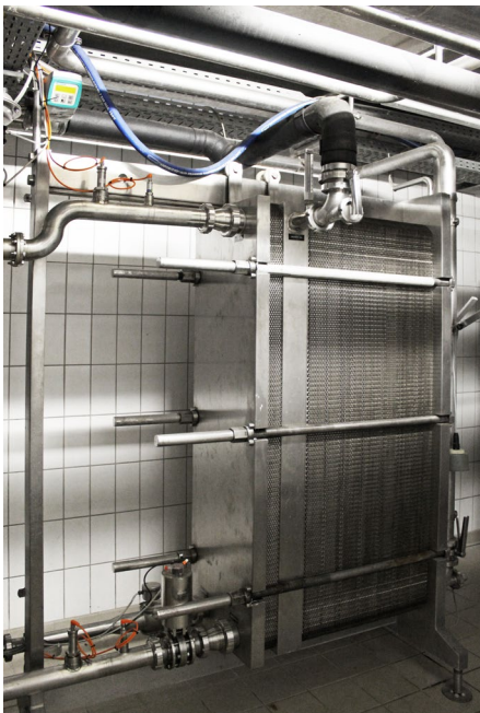
Glycol plate heat exchanger with TS temperature sensor and P41 pressure transmitter in the supply and return lines
