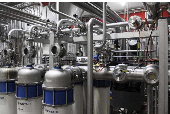
Crossflow membrane filtration with FTS flow monitor and TS temperature sensor
